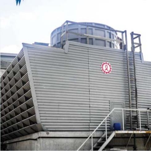
Project : Internation Industrial Limited LHC-453D-C2, 44-32-29 °C, 800 M 3 /Hr./Set
