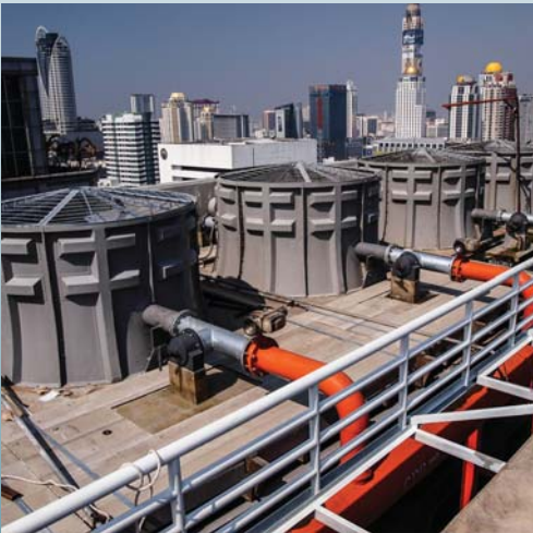
Project : Ploen Chit Building (BBTV) LHC-369D-C6, 38-32-28 °C, 1,536 M 3 /Hr./Set
