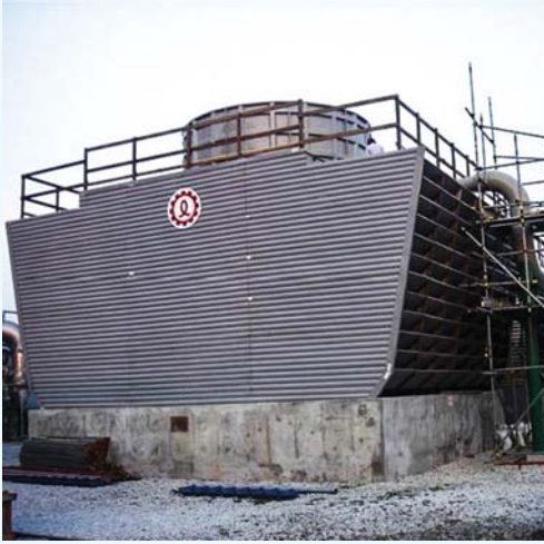
Project : Thai Plastic Line 5 LHC-475SD-C1 35.5-32-28.5 °C 1,100 M 3 /Hr./Set
