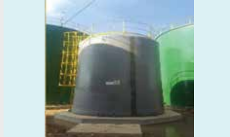
LOCATION : SARABURI POWER PLANT MODEL : LCT-V-60 m 3 x 2 SETS
