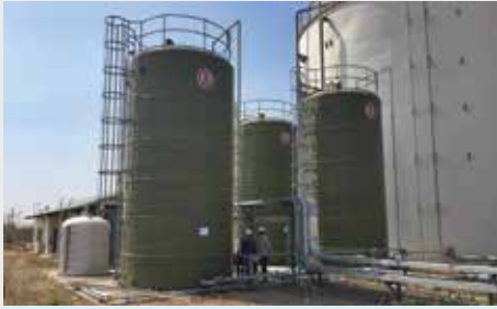
LOCATION : KNM PROJECT (THAILAND), CHACHOENGSAO MODEL : LCT-V-80 m 3 x 3 SETS
